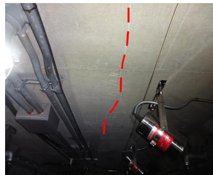
Sta.920~940m Type ① 균열 0.1/2.0
