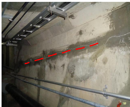
Sta.760~780m Type ② 균열 0.1/5.8
